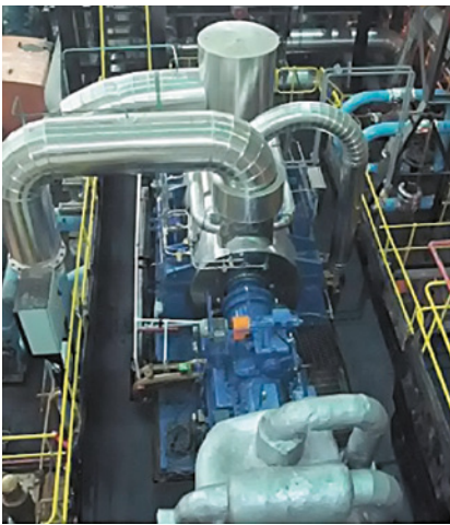
The Sulzer retrofitted installation
